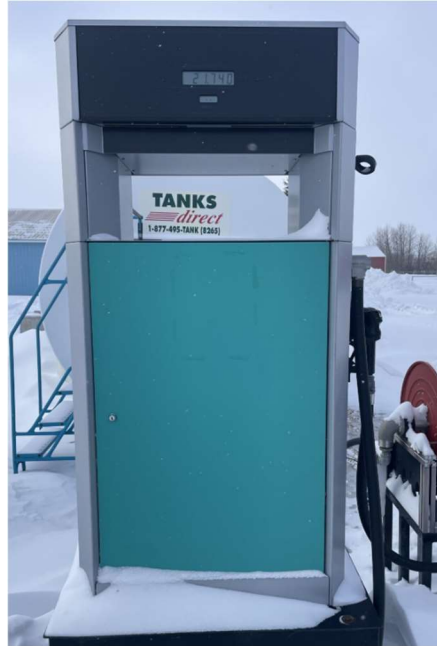
Image 6: View of Dispenser Cabinet
