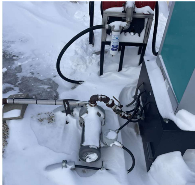
Image 3: View of AVGAS Transfer Pump
