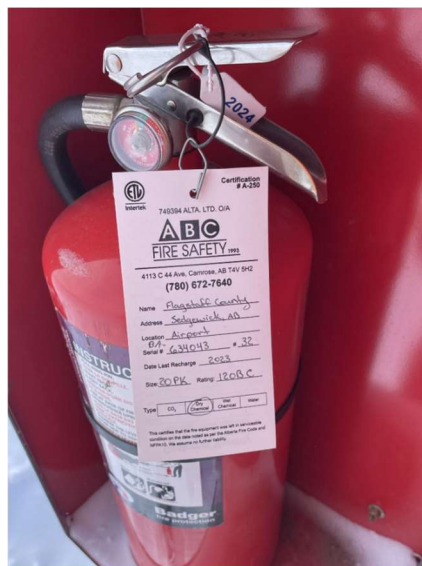
Image 5: View of Fire Extinguisher
