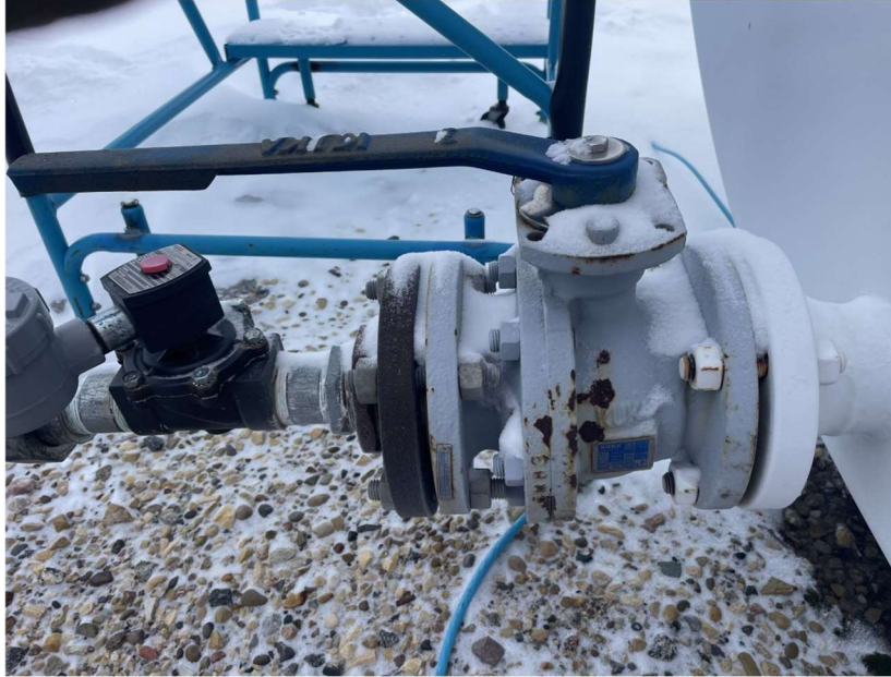
Image 10: View of piping penetrating secondary containment of tank
